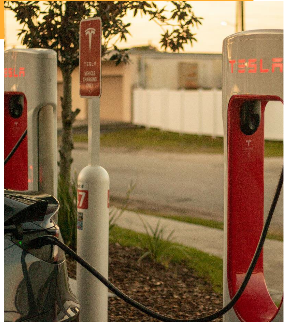
Charging Station Credit: Ryan Casburn, Kittelson & Associates, Inc.
