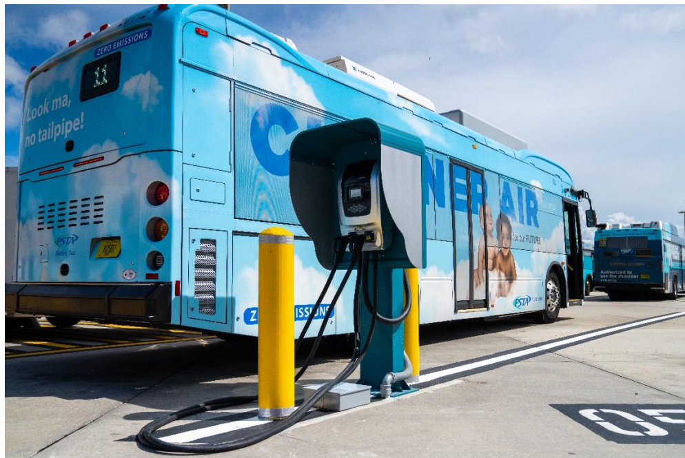
“Electric Bus Charging Station. Photo Credit: PSTA”
