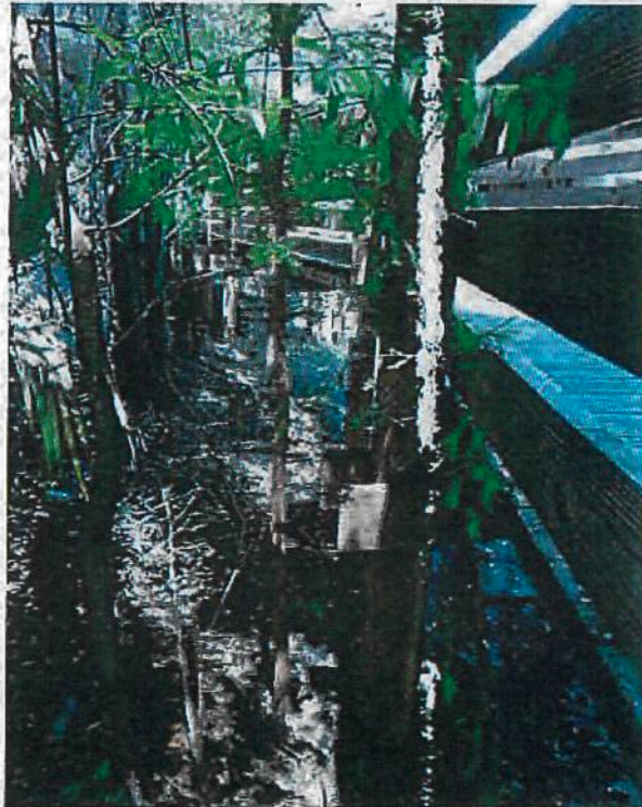
Photo 2. Subtle scarp from wave action underneath boardwalk
