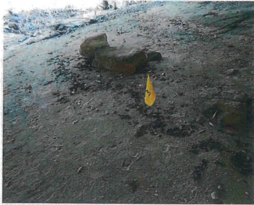
Photo 3. Debris line under Fletcher Avenue Bridge
