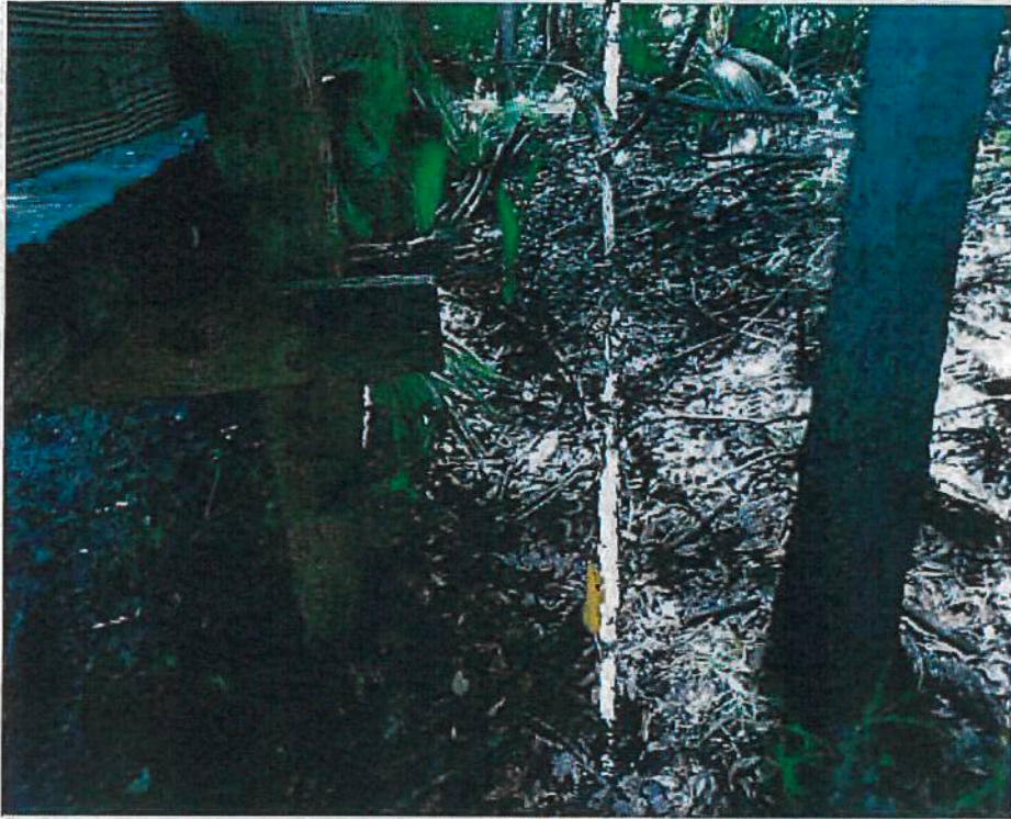
Photo 1. Boardwalk plus pin flag line marker at Hillsborough River/Morris Bridge Road Bridge
