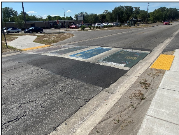
Marked Crossing at Shaw Elementary School and Regency Square Apartments was installed a few years ago and needs maintenance
