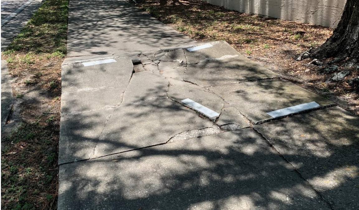
Cracked Sidewalk along the north side of Fletcher Avenue
