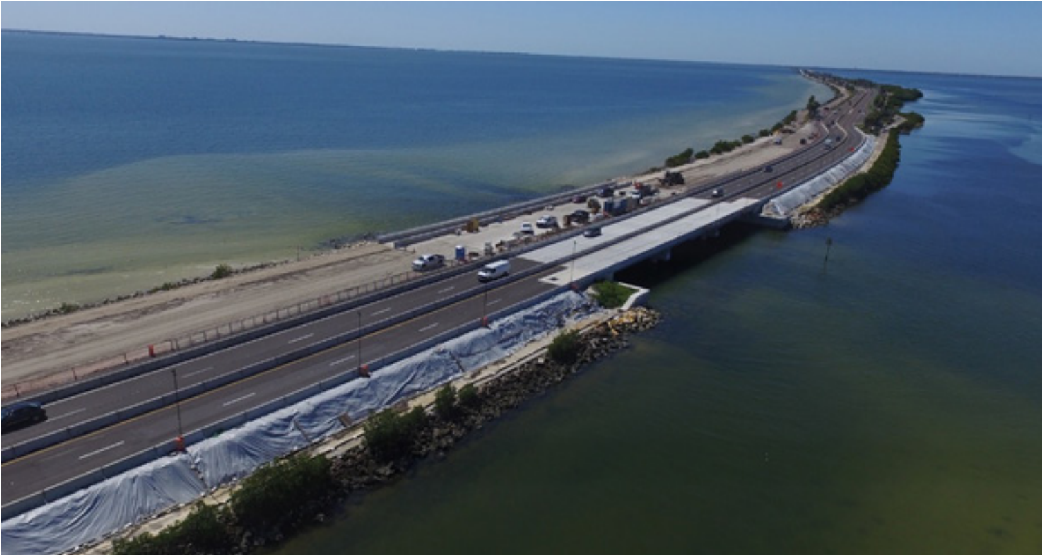
A portion of the Courtney Campbell Causeway is currently being reconstructed to create a channel through the bridge. This will improve circulation in Tampa Bay and improve water quality. The project will be completed before the end of 2019.
