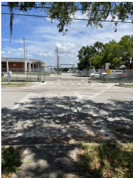
Image 60: Faded Crosswalks at with Exposed Brick at Entrance to Just
