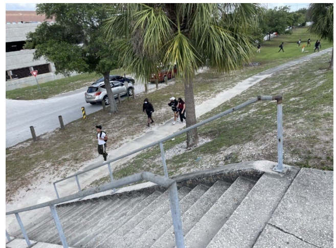
Image 61: Sand on Sidewalk and no ADA Ramp
