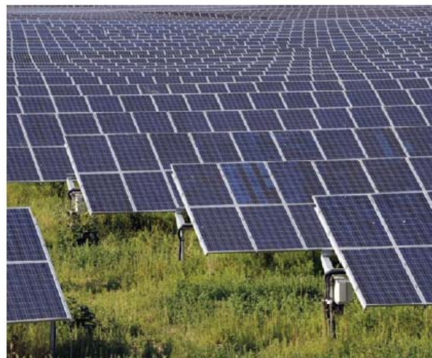
Solar panel field
