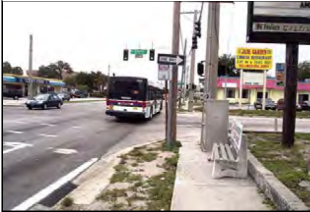
Figure 3-3 Example of Sidewalk Obstructed by Utilities
