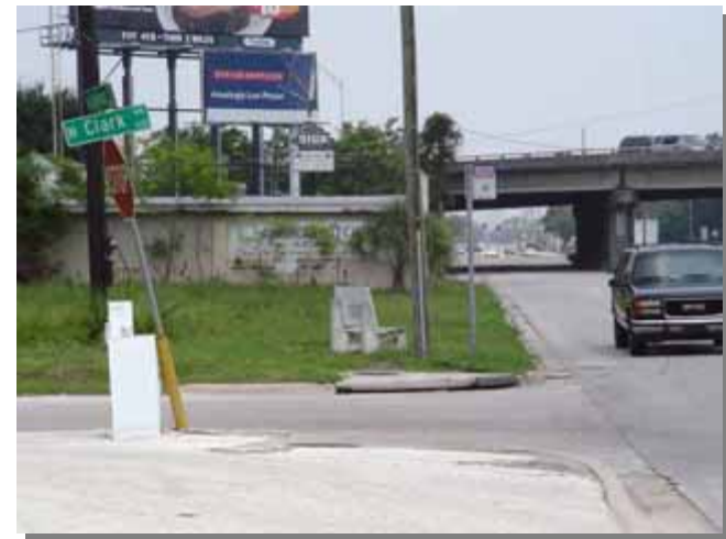
Figure 2.33: Unfortunately, many transit facilities are not - this stop is not located directly adjacent to a sidewalk and the existing curb does not have curb cuts.
